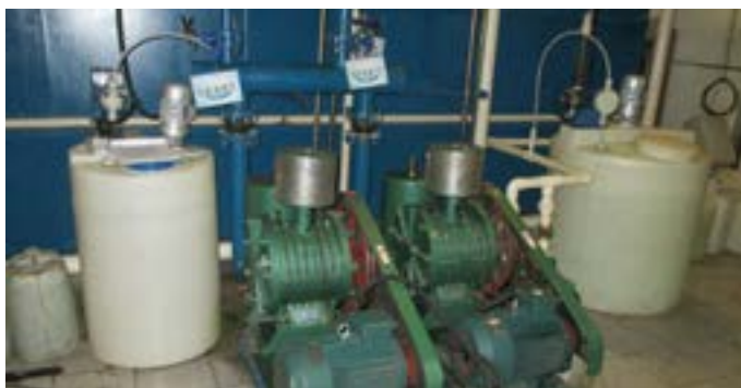
Membrane Recycled Water Treatment System
